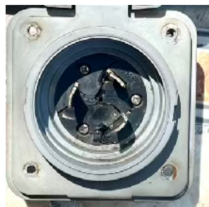
Streetside Power Inlet
