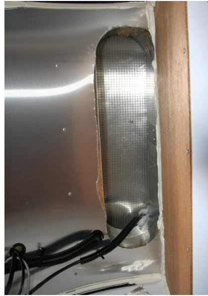
2: PV Panel Wire Through Refrigerator Roof Vent
